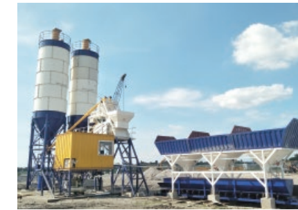
HZS50 batching plant
